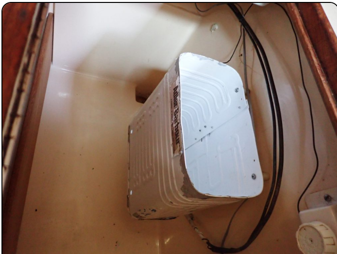
Fridge evaporator and control
