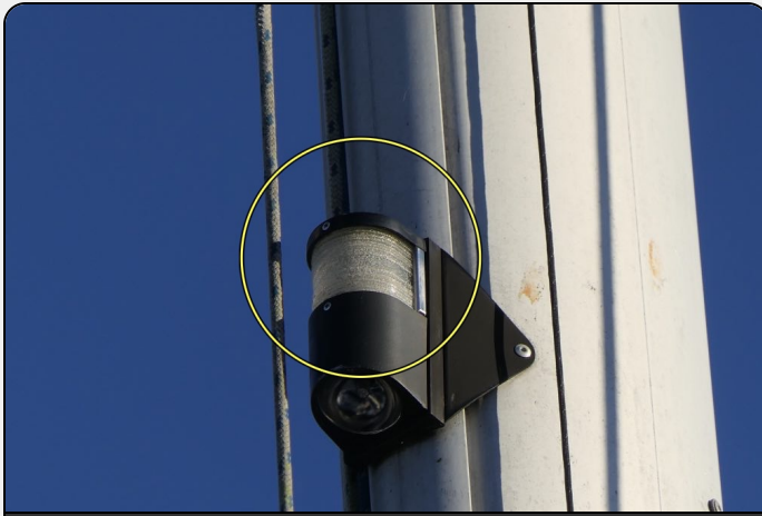
Check lamp in Masthead light
