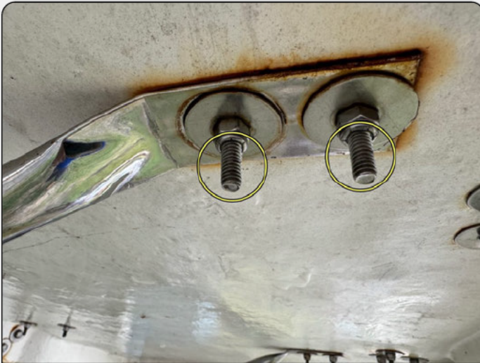
Bolts could pose a hazard and should be shortened or covered.
