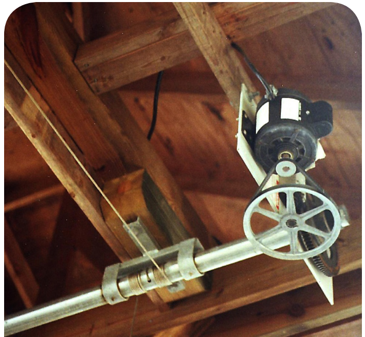
Photo 5. An image of the lift motor mounted on a metal plate, attached to the metal rod with the metal wires that are attached to the metal lift rods in Photo 2.
