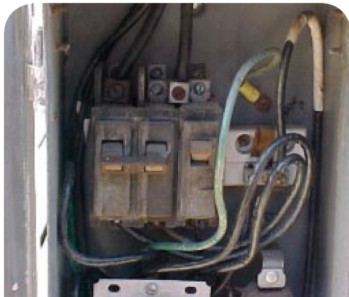
The grounding system in this dockside service panel was called into question in the investigation.
